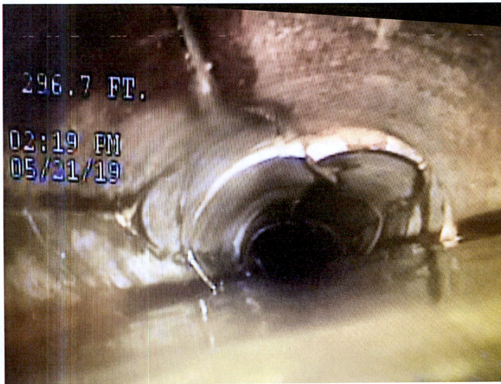
Clay Sewer Main with broken pipe, severely deformed, likely to collapse.
