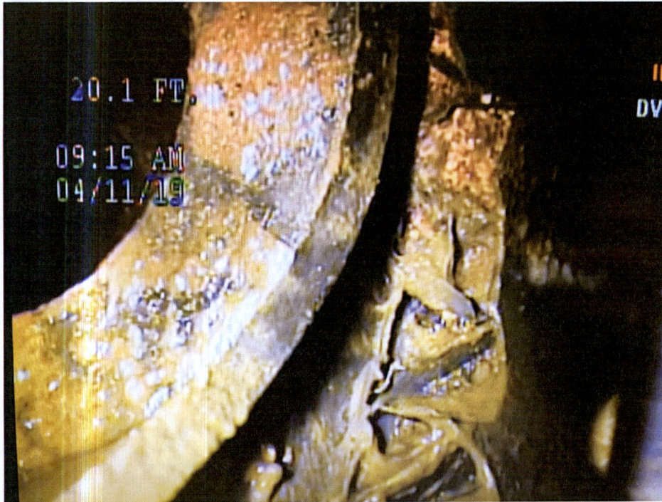
Service Line Tap into Truss pipe sewer Main, note the gap and failure to seal the joint
