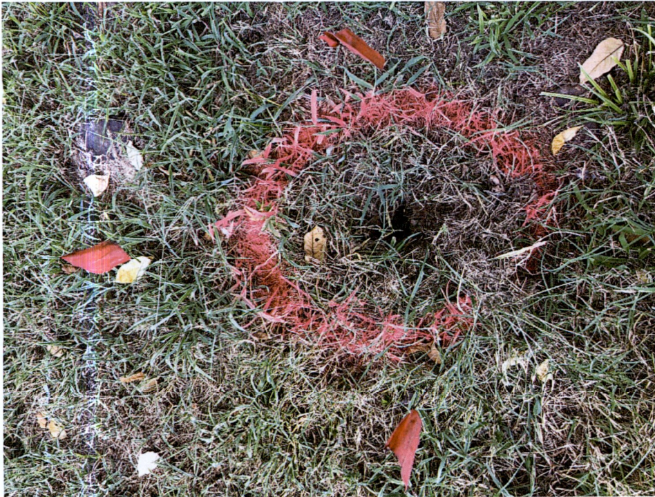
Private Service Line leaks that will require additional effort for repair.
